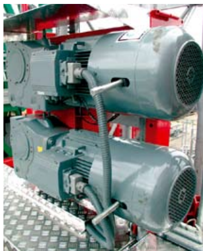
• Top drive unit on the roof
